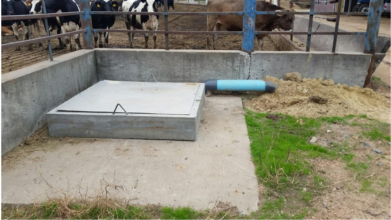
Figure 7: Manure tank pump-out riser to prevent manure overflow (after in Oct. 2016)
