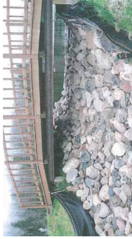
Above: This is a typical rip-rap rock chute dam for a high head. The steel sheet pile can be seen under the bridge. This dam will look very natural and in keeping with
