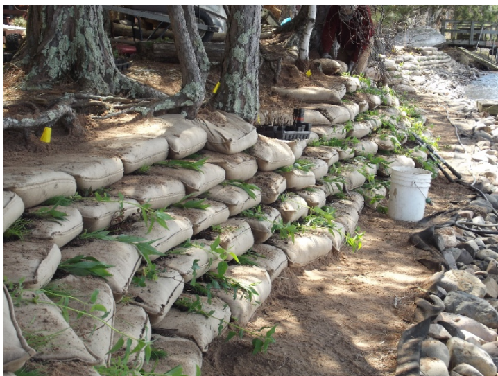
Installation of the rock rip rap and EnviroLok bag system in May 2017. Photos by Gary Pulford.
