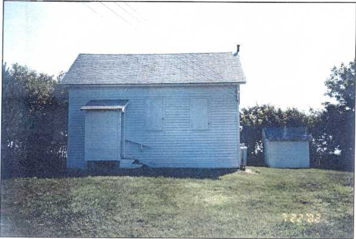
Kippenhan School on County Road MM first shown on 1906 Map. Used as Mead Town Hall until 1989. Currently a hunting camp.
