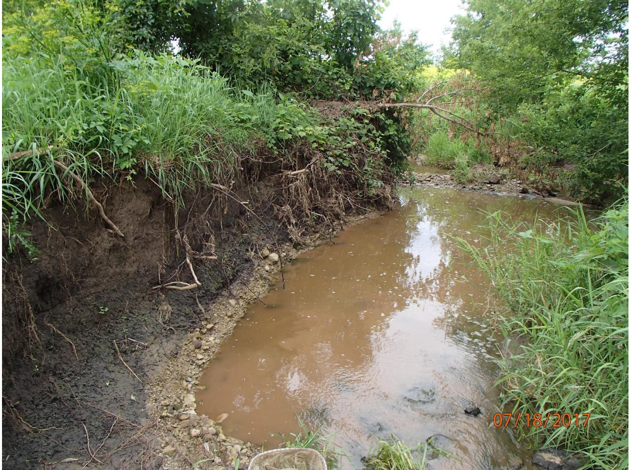
Photo 3: Streambank erosion along Pipe Creek upstream of Hwy 151. Photo taken by D. Bolha on July 18 th , 2017.
