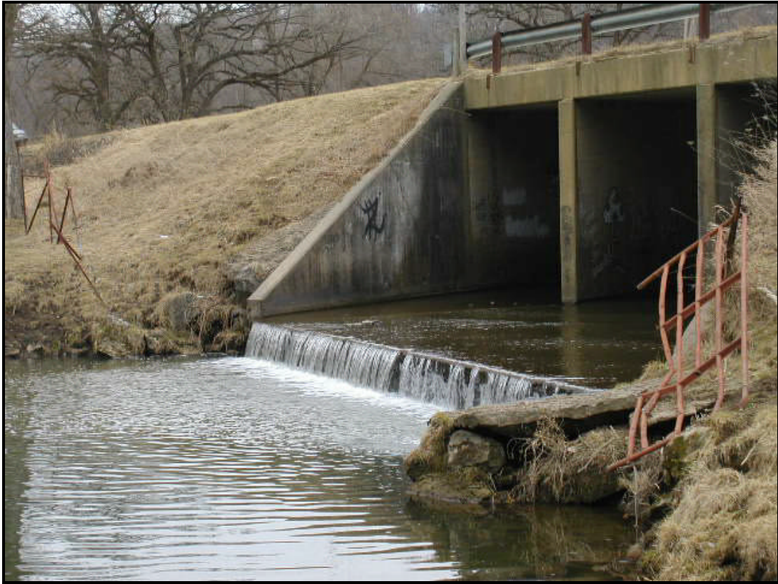
Figure A-7. Oversized culvert at confluence of Snowden Branch and French Creek
