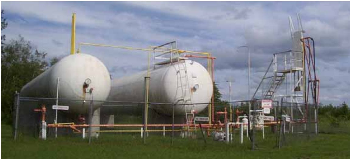
Storage tanks and gas lines provide economic development opportunities.
