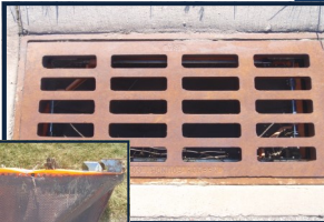
Protection device sits in drain
