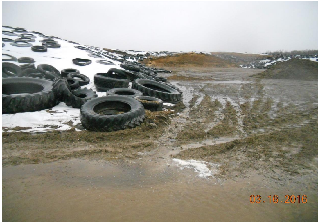
Leachate Running off of feed pad, on to driveway. Feed sitting in water.
