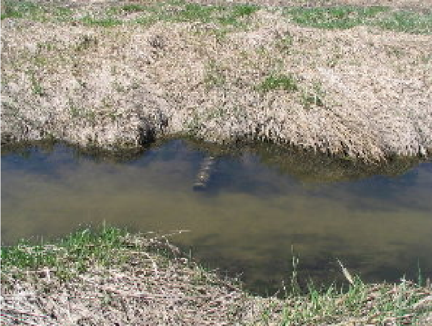
Figure 17. Daintile to Parsons Creek. This submerged daintile was observed (along with many others) in the ditched Main Stem of Parsons Creek near the confluence with the Wetland Tributary. April 14, 2006.
