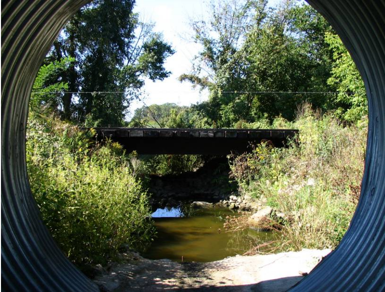
Figure 22. Parsons Creek East Tributary feeder below the railroad track culvert looking downstream from inside the culvert. The probe was attached to a rerod at the base of the concrete that can be seen at the bottom of this photo (Sept. 14, 2005)
