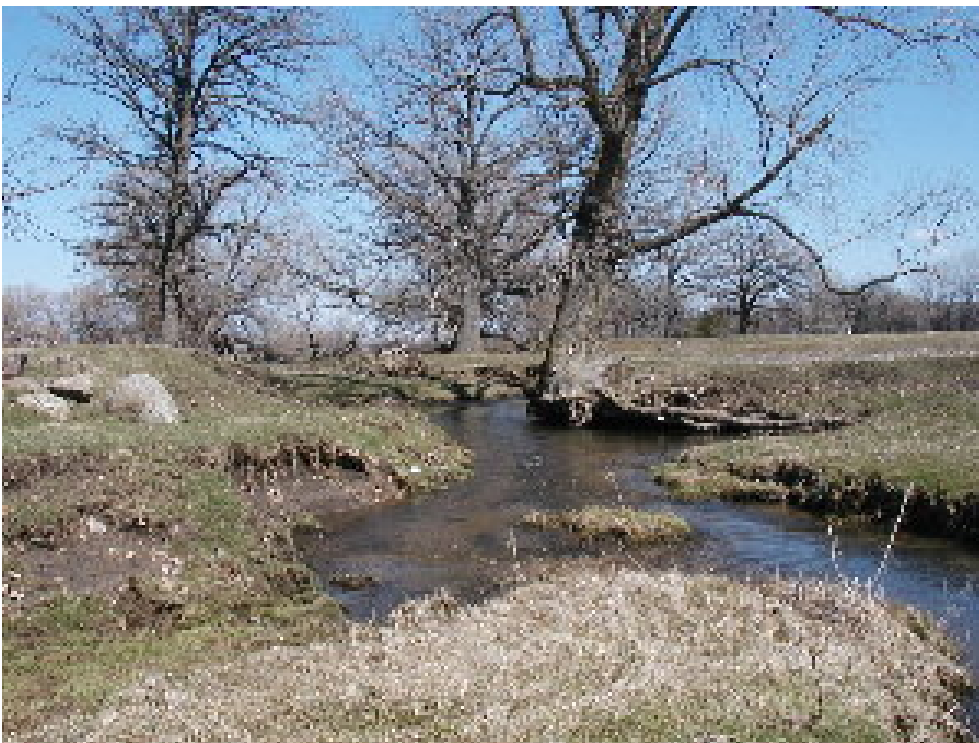
Figure 21. Parsons Creek erosion problems below HWY B. April 1, 2004.
