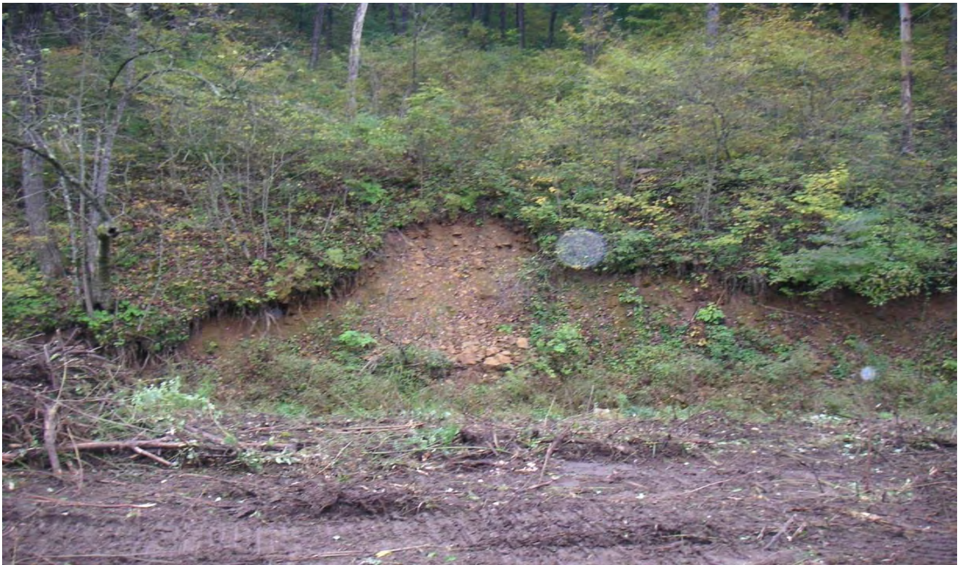
The stream impinged on the hillside because of a high bank on the opposite side causing substantial erosion. Tapering this high bank should slow stream velocity during a high water event, easing erosion on the hill.
