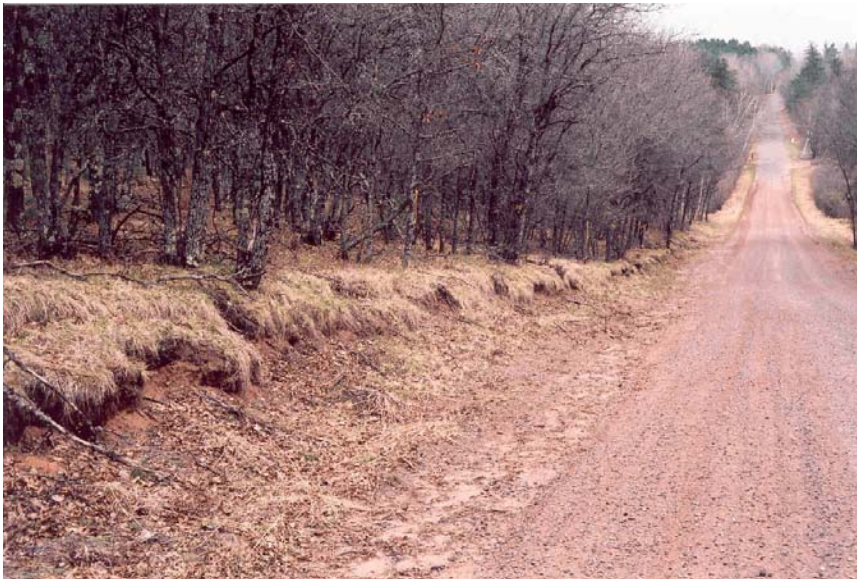
Figure 22. Potential sediment sources to the Kimball Lakes comes from road shoulders.
