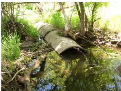
19- ABANDONED CULVERT COCO CREEK (RM 4.37)
