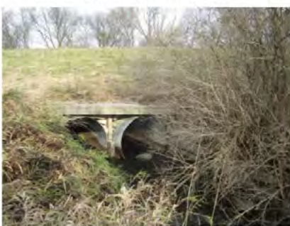
23- CTH KF (RYAN ROAD) COCO CREEK TRIBUTARY (RM 1.34)
