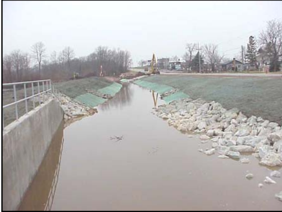
Figure 9. Picture of the rerouted stream with the berm between the stream and the lake on the left and HWY 151 on the right.
