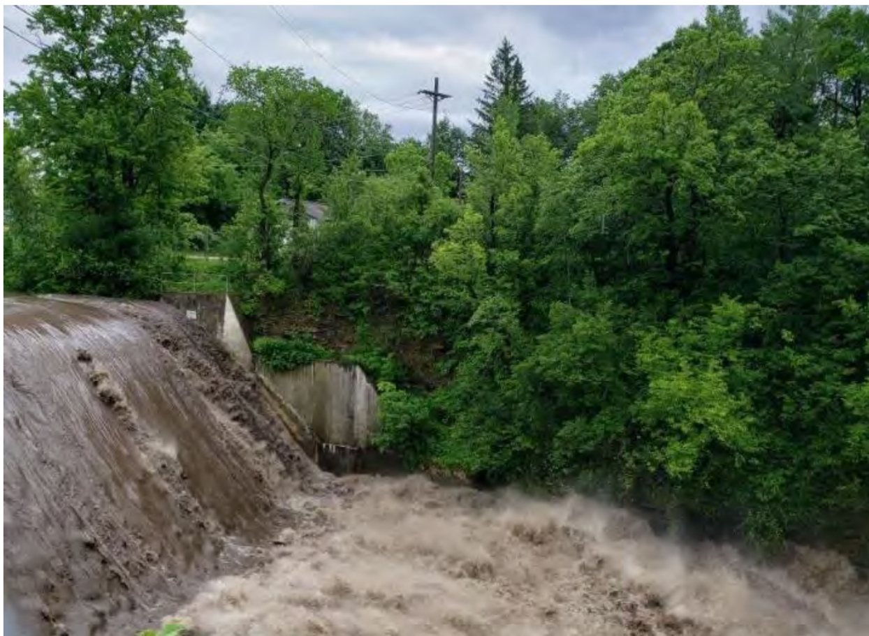
Figure 3. June 29, 2020 Flood at Junction Falls
