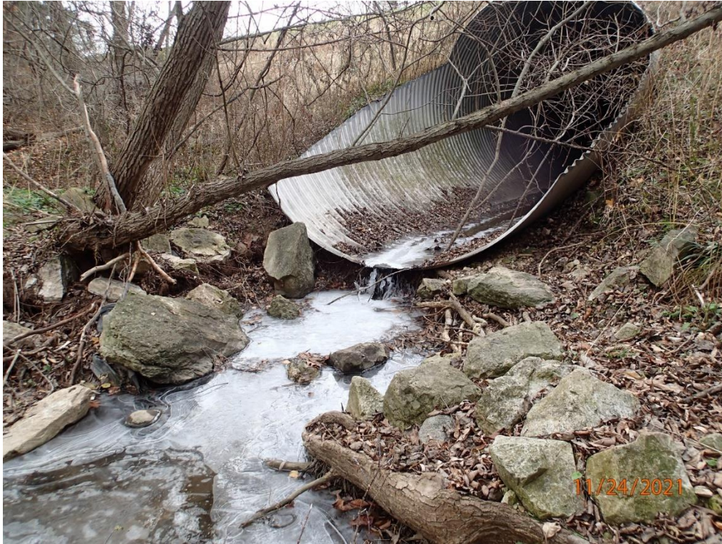
Site #4. WBIC 3000159 Perched culvert east side of CTH R
