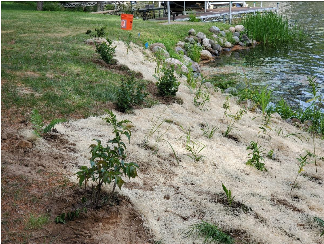
Figure 24. Photos taken 6-30-22 of the completed shoreland habitat restoration project. Photo credit Stephanie Boismenu
