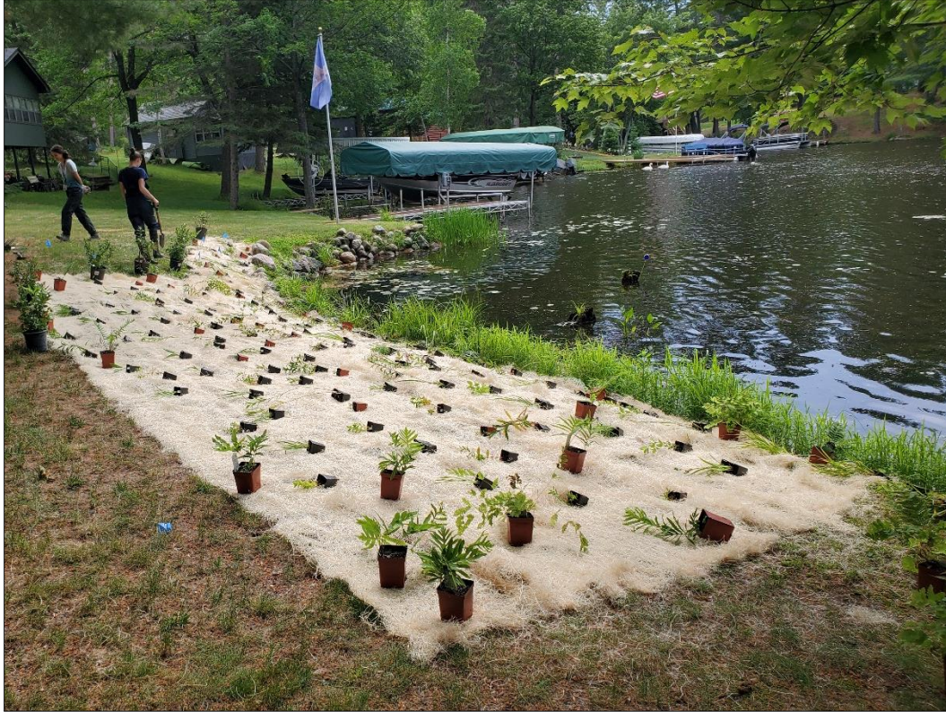
Figure 19. Photos taken 6-30-22 showing the progression of the shoreland habitat restoration project. Photo credit Stephanie Boismenu
