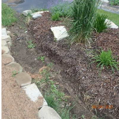
Photo 2: From the neighboring property, the runoff is forming gullies on its way to the lake.
