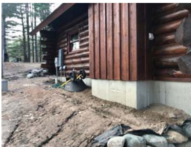
Photo 2: Infiltration South Side Before May 2019
