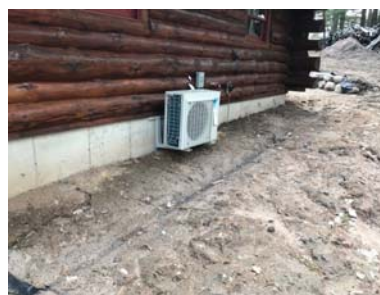
Photo 3: Infiltration North Side Before May 2019
