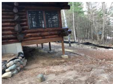
Photo 1: Infiltration South side Before May 2019
