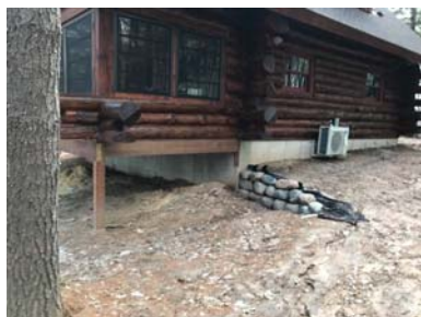
Photo 4: Infiltration North Side Before May 2019
