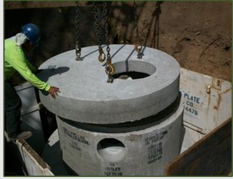
Oil grit separator
