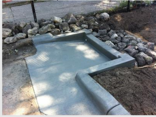
Custom Concrete Forebays
