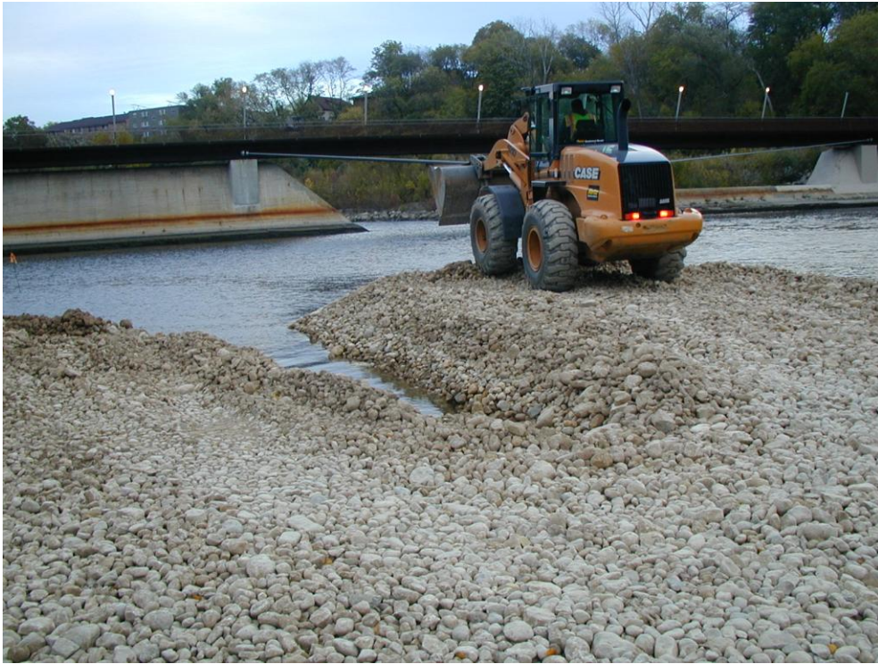
Photo 5. Approaching the limits of the causeway construction. “Rust” line along the former North Avenue Dam spillway is the 1997 high water mark of Lake Michigan approximately 3.5-ft above current lake elevation.
