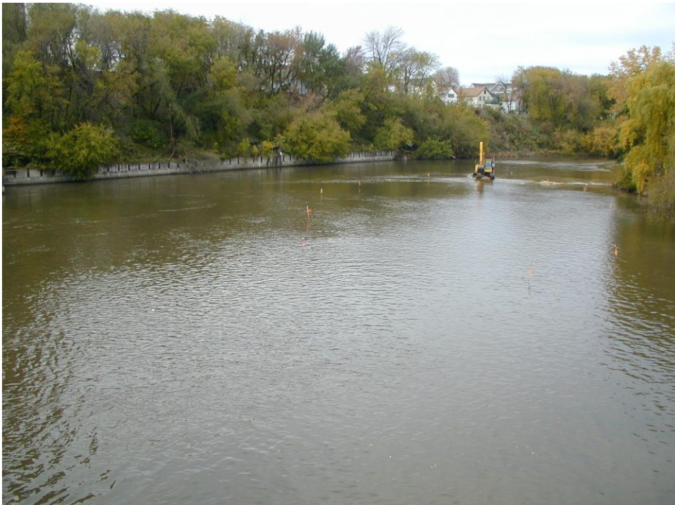
Photo 6. Excavator backing off the temporary causeway following redistributing the causeway as reef material. Orange flag tape and rebar outline the limits of the former causeway.
