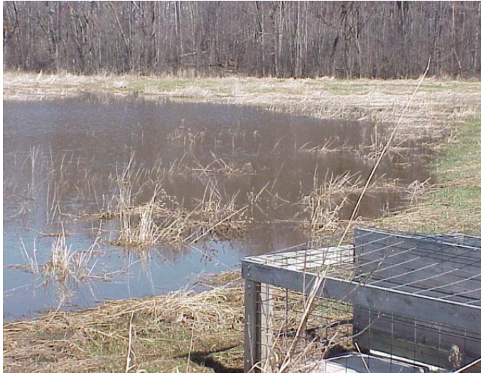
Basin and outlet trash rack
