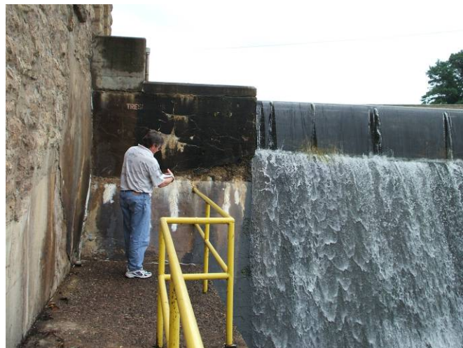
A WDNR dam safety engineer inspects the Neshonoc Dam on the LaCrosse River
