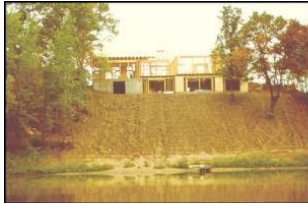
Denuded shoreland at a new construction site
