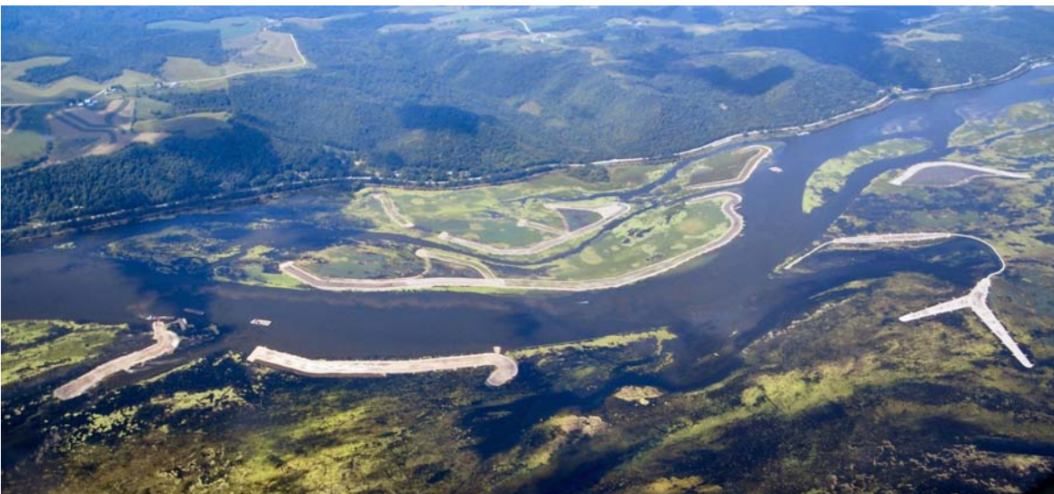
Photo 1. Construction of Pool 8 Islands, Phase III, on the Mississippi River south of La Crosse, WI. The view is looking west towards Minnesota along a secondary side channel (Raft Channel) of the Mississippi. Photo courtesy of USGS-Upper Midwest Environmental Sciences Center, La Crosse, WI.
