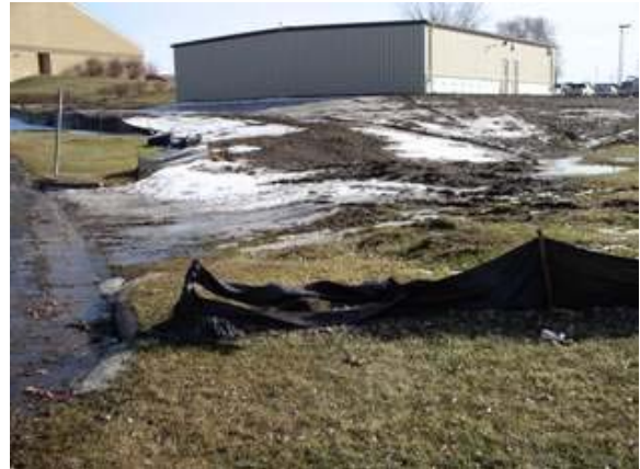
Construction site erosion, Dunn County.
