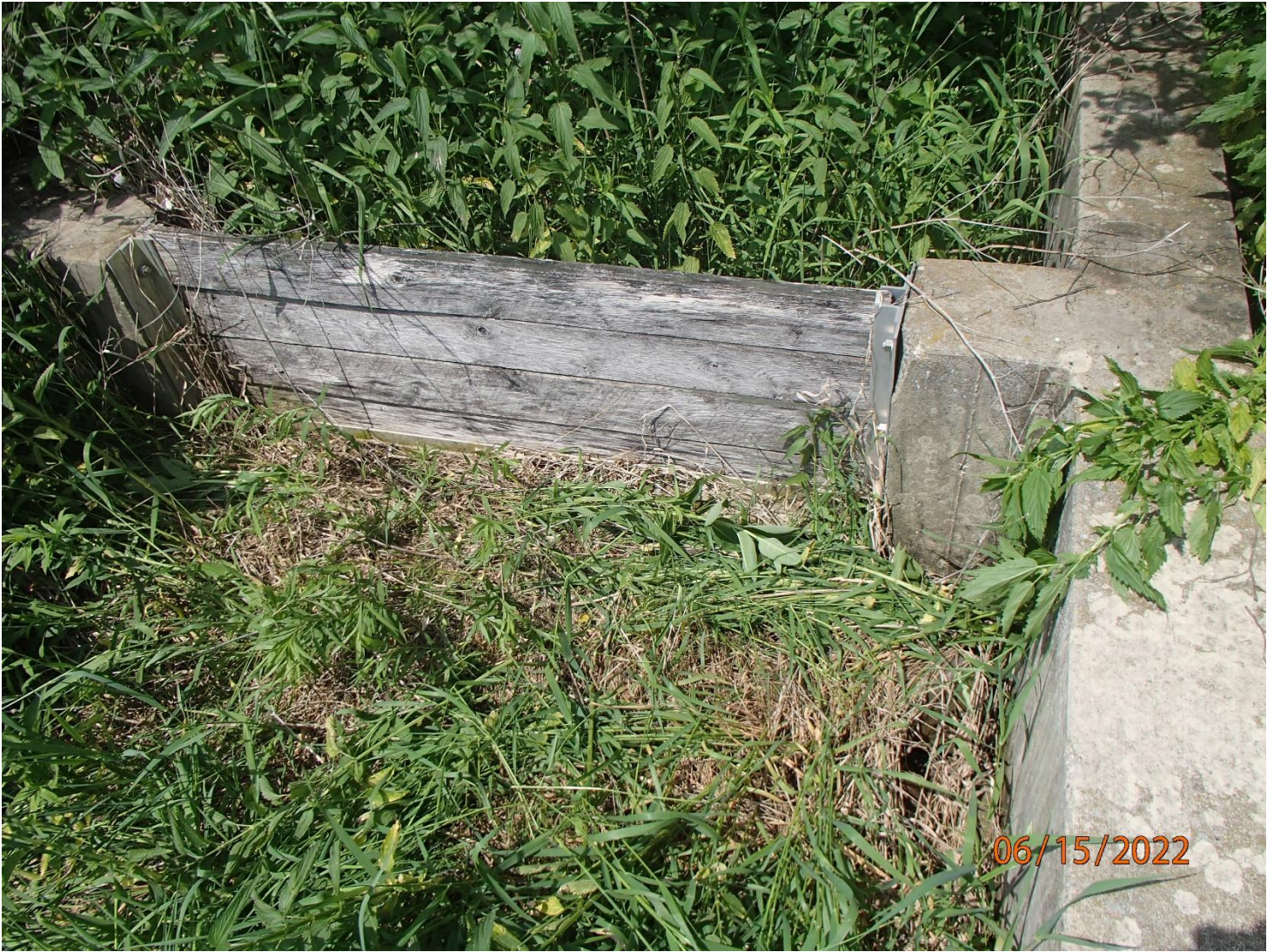
Photo 2: Packwaukee Sanitary District No. 1 Outfall Water Control Structure. Photo taken by David Bolha on 6/15/2022.
