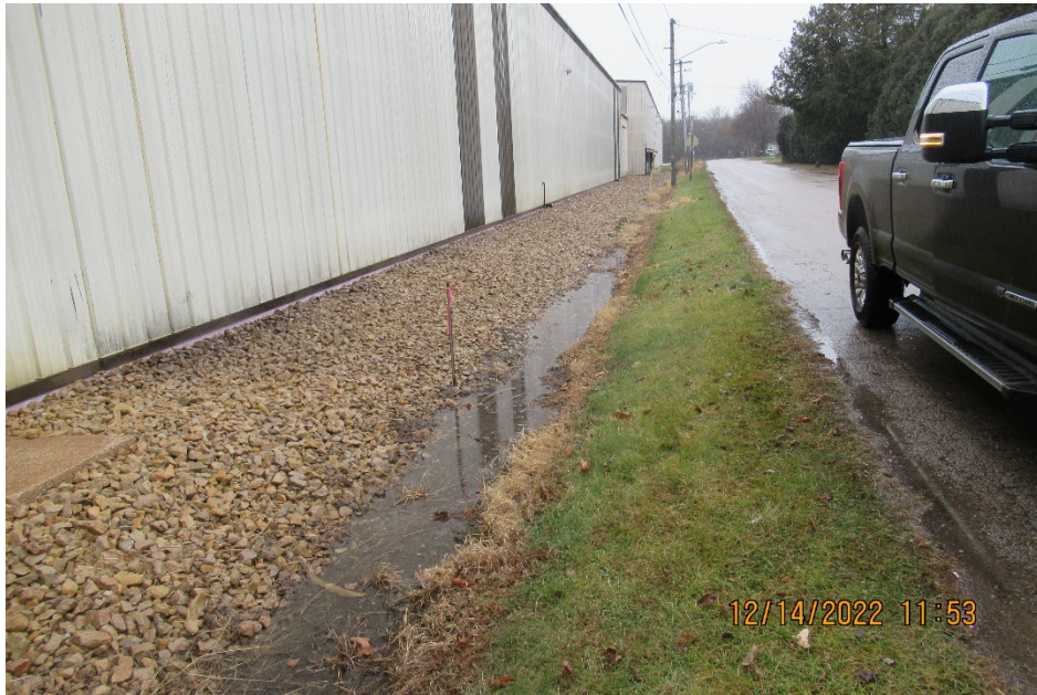
Drainage Ditch w/Standing Stormwater – South
