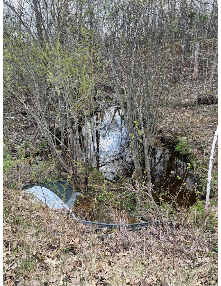
Photo 8. Unnamed Tributary at 17 th Avenue looking downstream.
