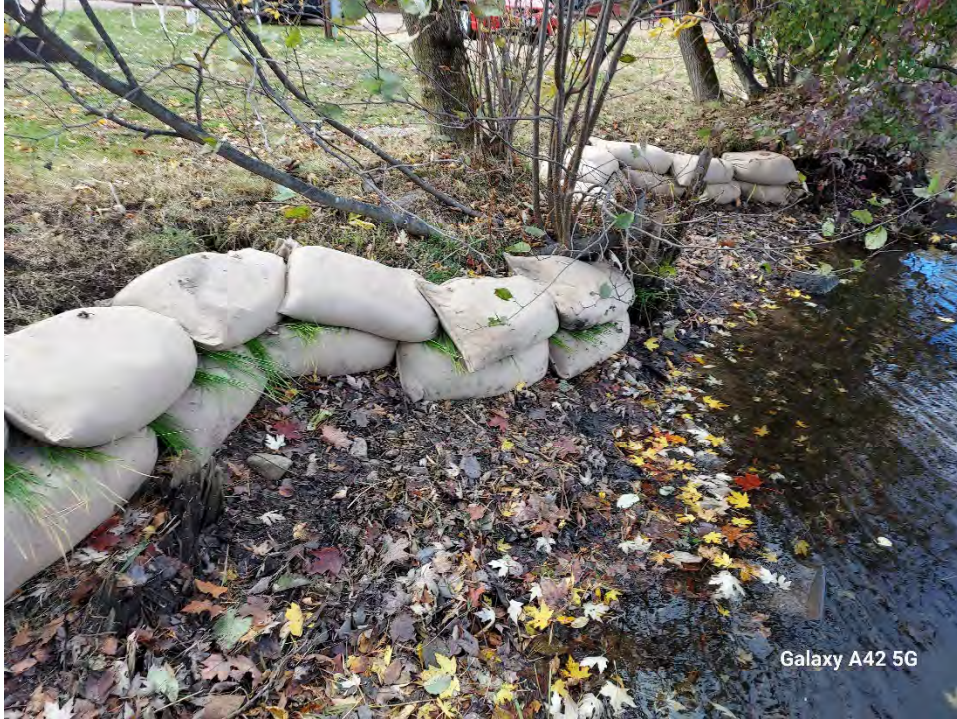
Photo 5: Second course installed. Did not put bags in front of woody vegetation unless needed. Majority of woody vegetation had good root structures holding soil in place.
