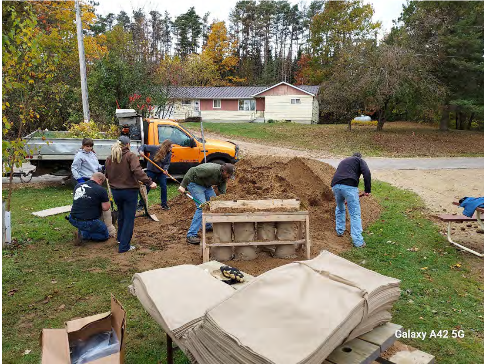
Photo 1: Showing bags being filled. Note no erosion control was used as the soil was placed in a depression and could not leave site.
