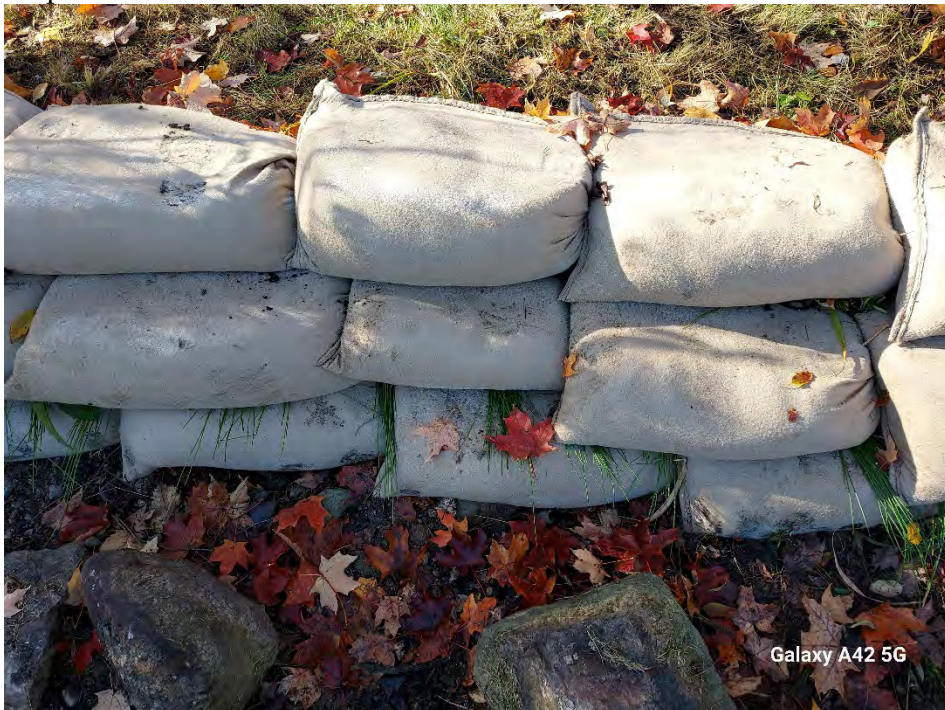
Photo 6: Third course installed, 2 connectors per bag and roughly 3 plants per bag. Different species of plants used in third row to accommodate less water.
