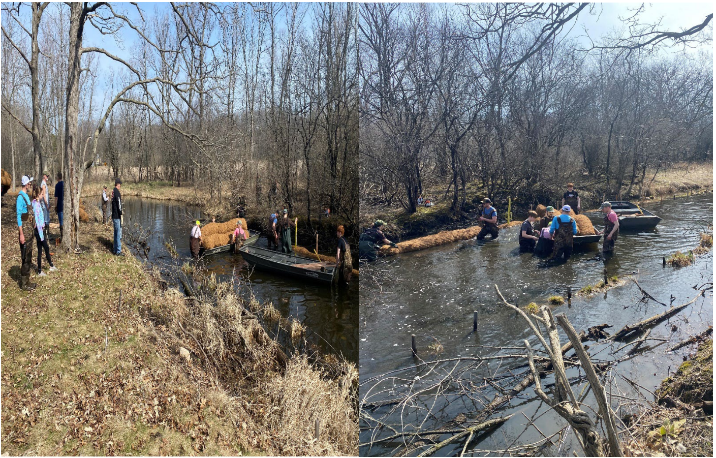
Row boats and chest waders were critical for getting materials to the “hard to reach” north side of the creek.
