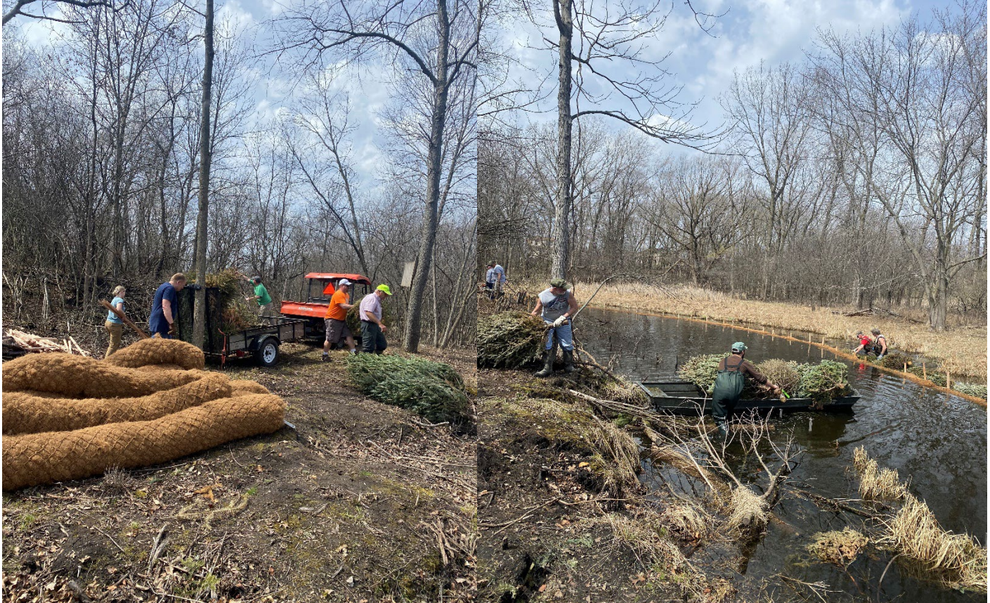
Recycled Christmas trees are added to the back side of the choir logs to trap the sediment and re-establish the banks
