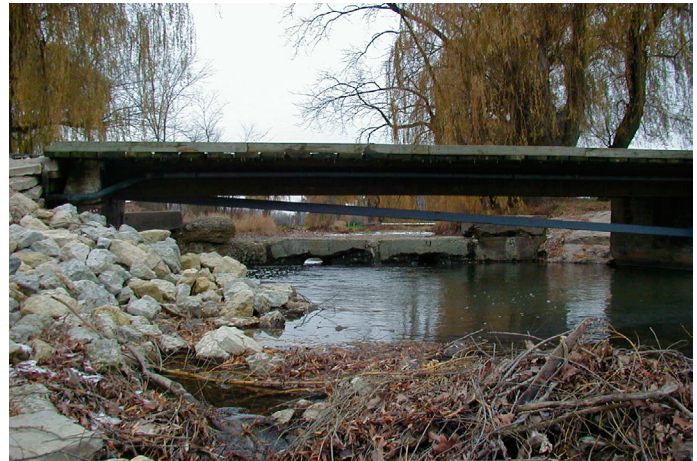
Before Restoration, Kenosha County Club Dam
