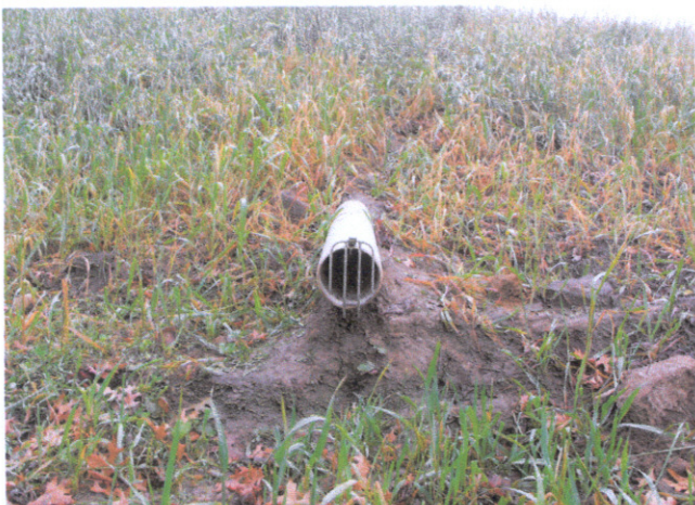
Outlet pipe with animal guard.
