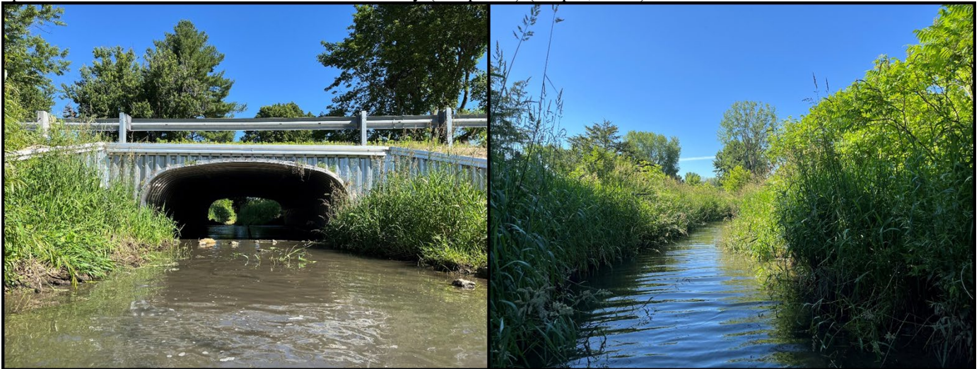
Photo 4. Improperly set culvert upstream of County Highway Y road crossing on Roxbury Creek. Right photo taken near the beginning of the fish survey on Roxbury Creek upstream of CTH Y. Roxbury Creek upstream of CTH Y near the end of the fish survey (left photo) (Map 3, dot 4).
