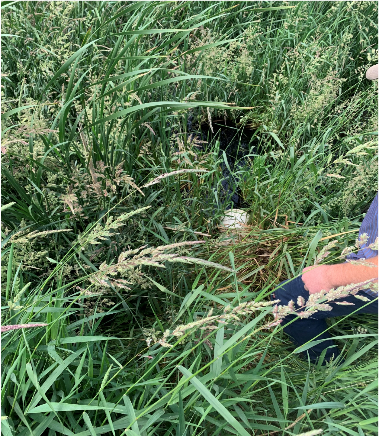
Photo 3: Discharge pipe into receiving wetland, with small pocket of standing water that diffuses further away from pipe.
