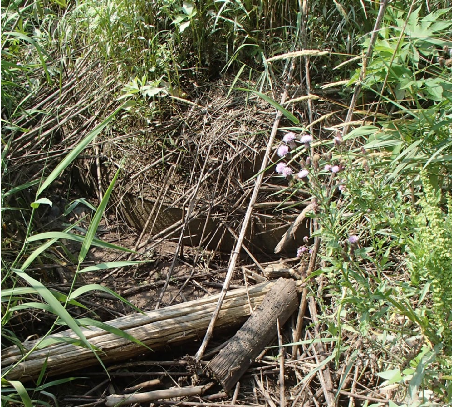
Photo 2: Manhole 7110. Photo taken by David Bolha on July 11 th , 2024.
