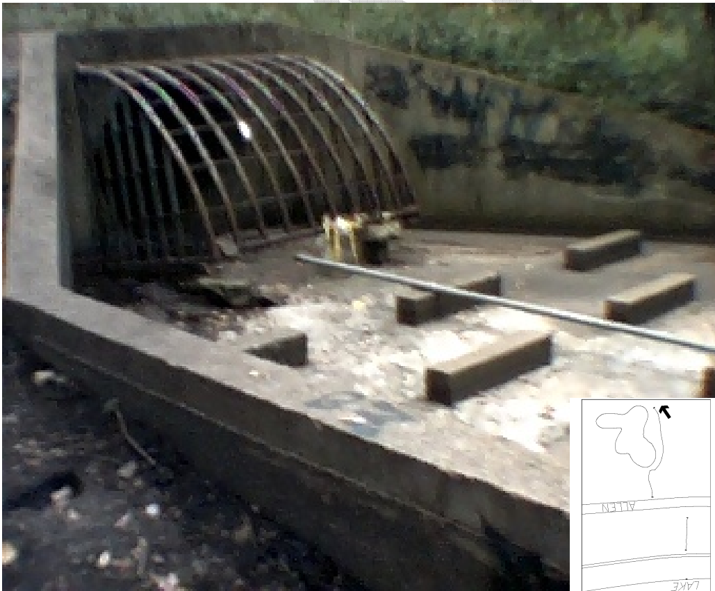
Figure 8- 54 inch Pipe Outfall at Park West
