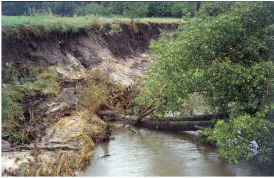
Streambank erosion before restoration
