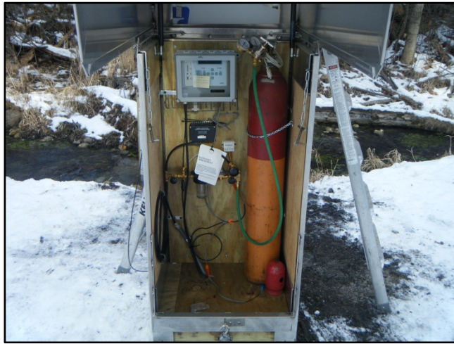
Nitrogen tank, pressure transducer, datalogger, and telemetry equipment inside the gaging station
