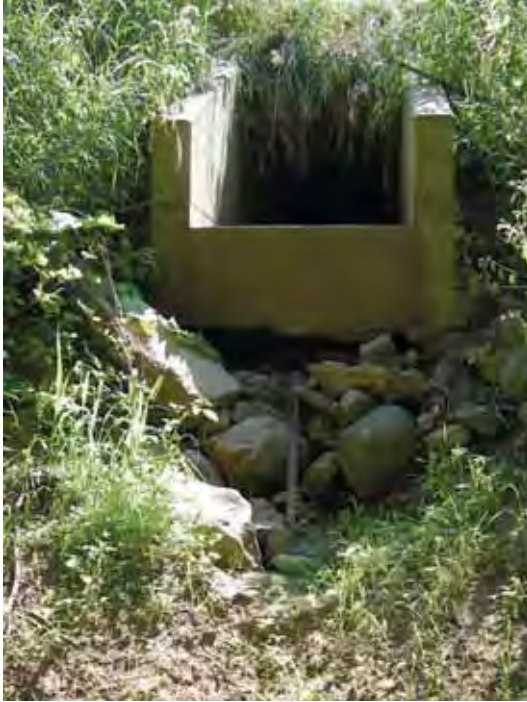
Figure 2-6. Eight-foot deep scour hole by a culvert in reach 8 of the West Branch (priority site E-4)
