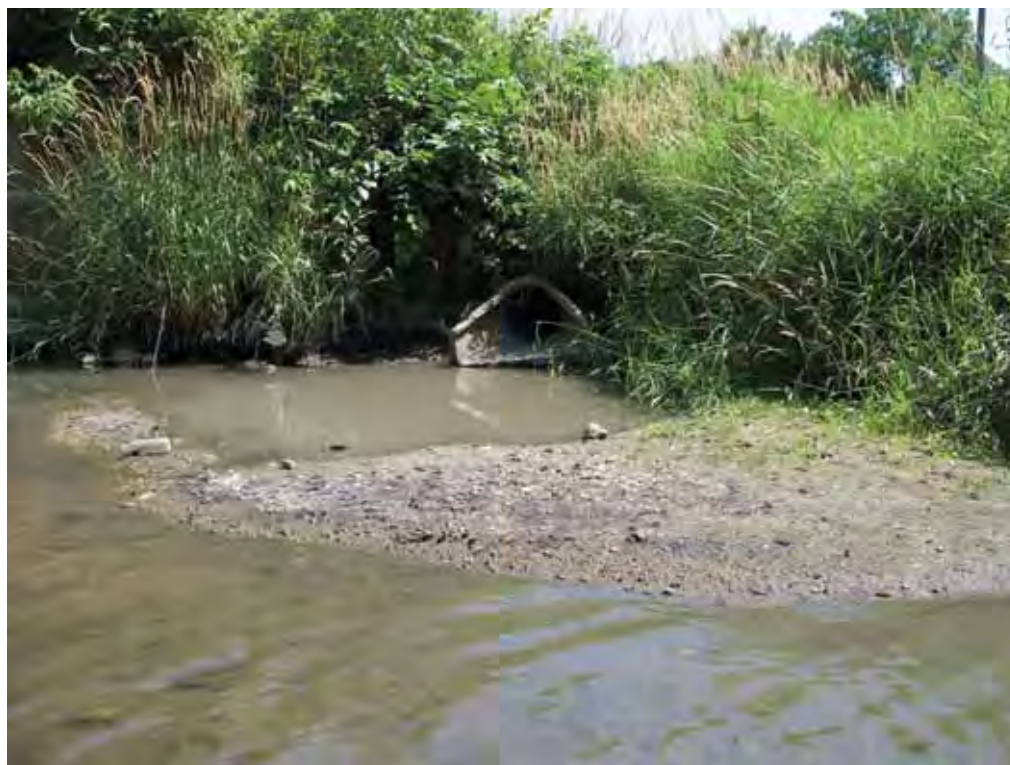
Figure 2-4. Priority site O-3, an example of an outlet with erosion problems due to high runoff volumes.
