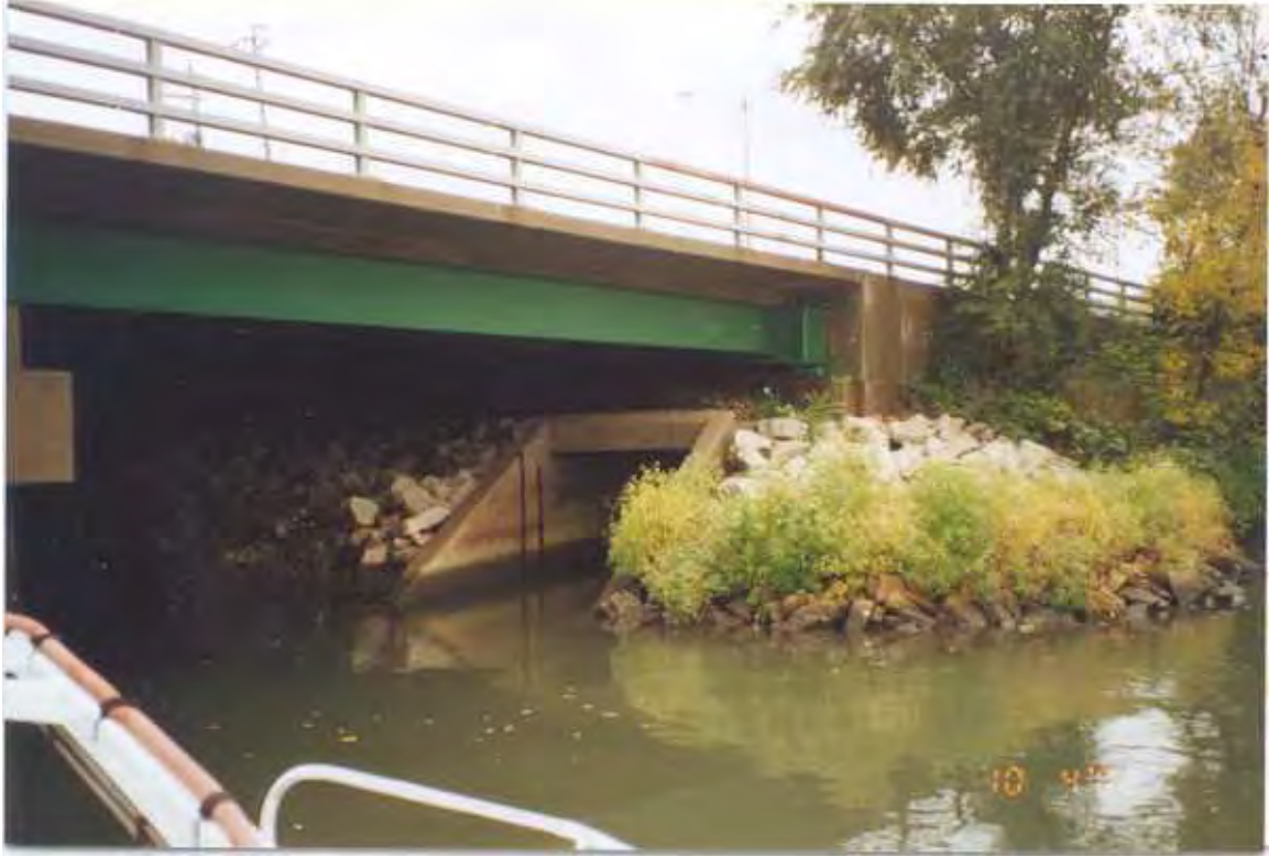
PHOTO 2 – October 4, 2002 – Kinnickinnic River Taken by Tor Hansen, Barr Engineering Left abutment Becher Street Bridge showing concrete box stormwater outlet. Taken from boat in river while looking southwest.
