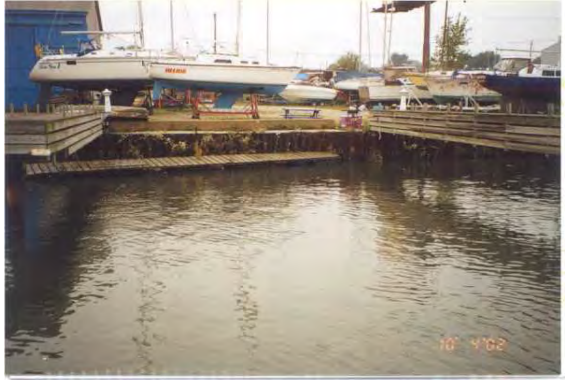
PHOTO 8 – October 4, 2002 – Kinnickinnic River Taken by Tor Hansen, Barr Engineering Steel sheet pile wall along Parcel 429. Looking west.
