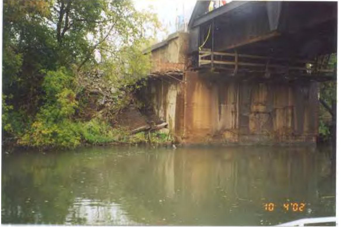
PHOTO 40 – October 4, 2002 – Kinnickinnic River Taken by Tor Hansen, Barr Engineering Railroad bridge abutment at downstream end of Parcel 425 downstream from photo 39. Looking north
