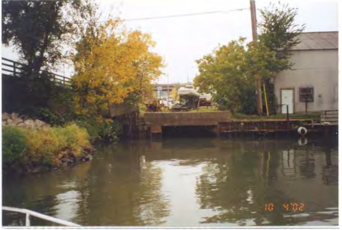
PHOTO 3 – October 4, 2002 – Kinnickinnic River Taken by Tor Hansen, Barr Engineering Concrete box stormwater outlet and upstream end of steel sheet pile wall along Parcel 429. Taken from boat looking west.
