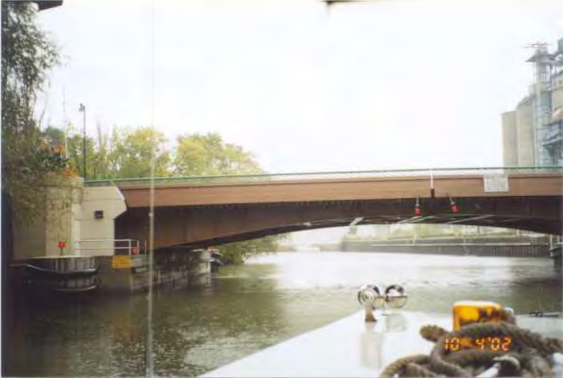
PHOTO 73 – October 4, 2002 – Kinnickinnic River Taken by Tor Hansen, Barr Engineering Upstream side of Kinnickinnic Avenue Bridge and left abutment. Looking east.
