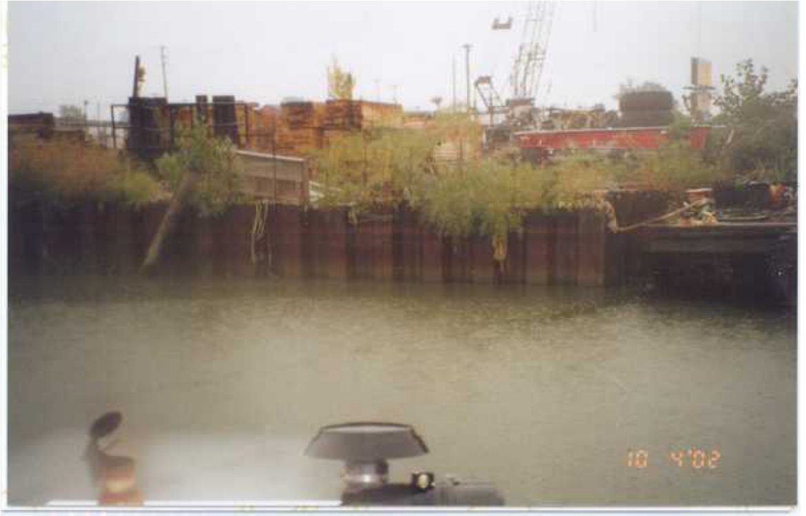
PHOTO 55 – October 4, 2002 – Kinnickinnic River Taken by Tor Hansen, Barr Engineering Steel sheet pile wall at corner of Parcel 433 where river turns from northerly flow to easterly flow. Looking south.
