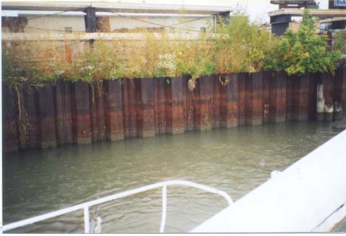
PHOTO 49 – October 4, 2002 – Kinnickinnic River Taken by Tor Hansen, Barr Engineering Steel sheet pile wall along Parcel 433. Looking east.
