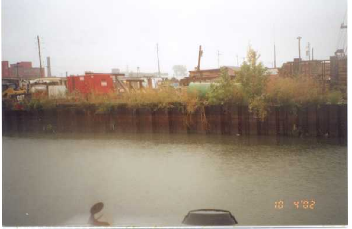
PHOTO 56 – October 4, 2002 – Kinnickinnic River Taken by Tor Hansen, Barr Engineering Steel sheet pile wall along Parcel 433. Looking south.
