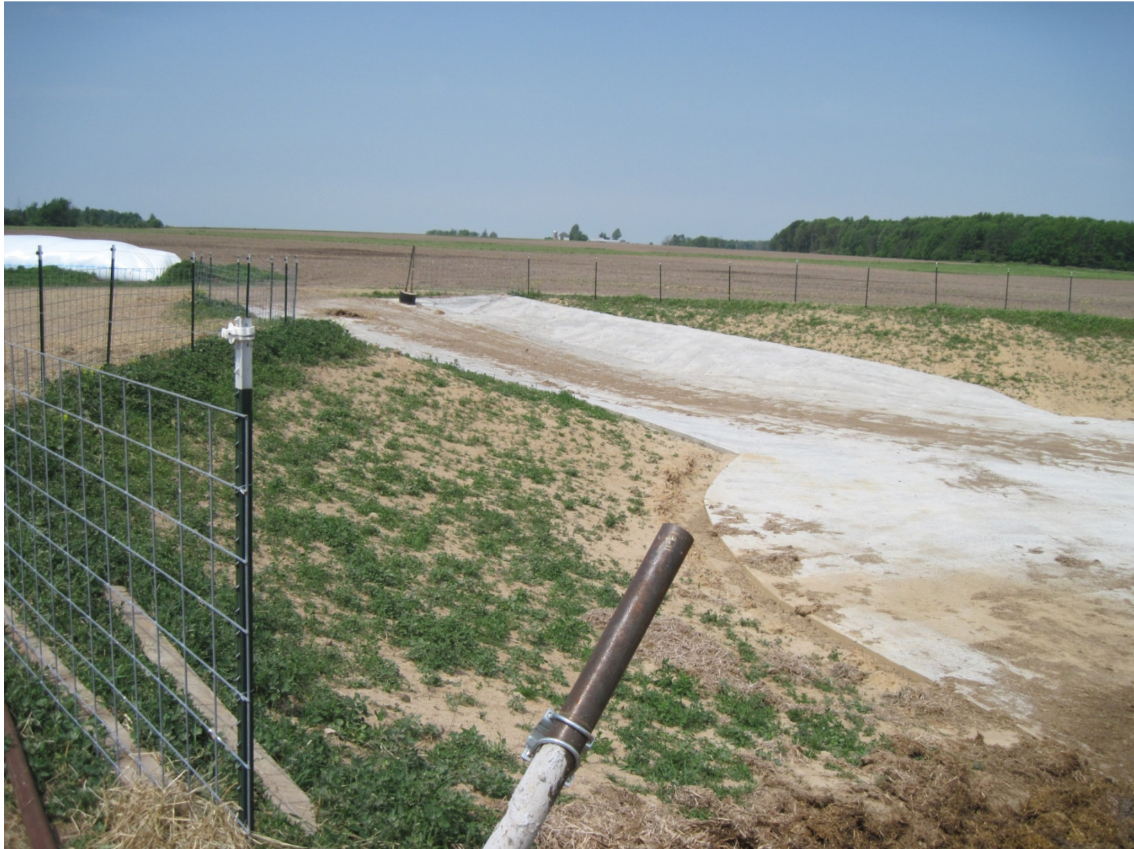
May 24, 2012 – This photo is taken standing on the feedlot push-off ramp, on the southeast side of the long term manure storage facility, looking to the west at the drive in ramp off the southwest corner of the manure storage facility. The floor of the facility is sloped from south to north, north being the deepest end of the facility. Fence is up and seeding on the dikes is just starting to come up. The push off bar will be installed when the level of the manure reaches the floor at the south end of the facility.
