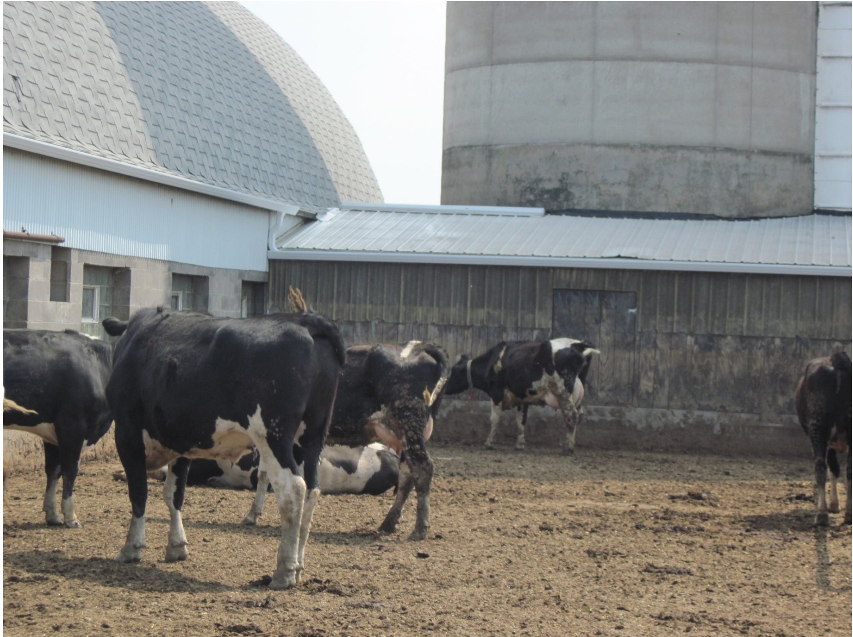
May 24, 2012 – Standing on the south side of the barn, on the feedlot, looking northeast at the gutters along the south side of the barn. Since this feedlot is in a SWQMA, all clean water needs to be diverted. Roof gutters were used to catch and divert clean water.
