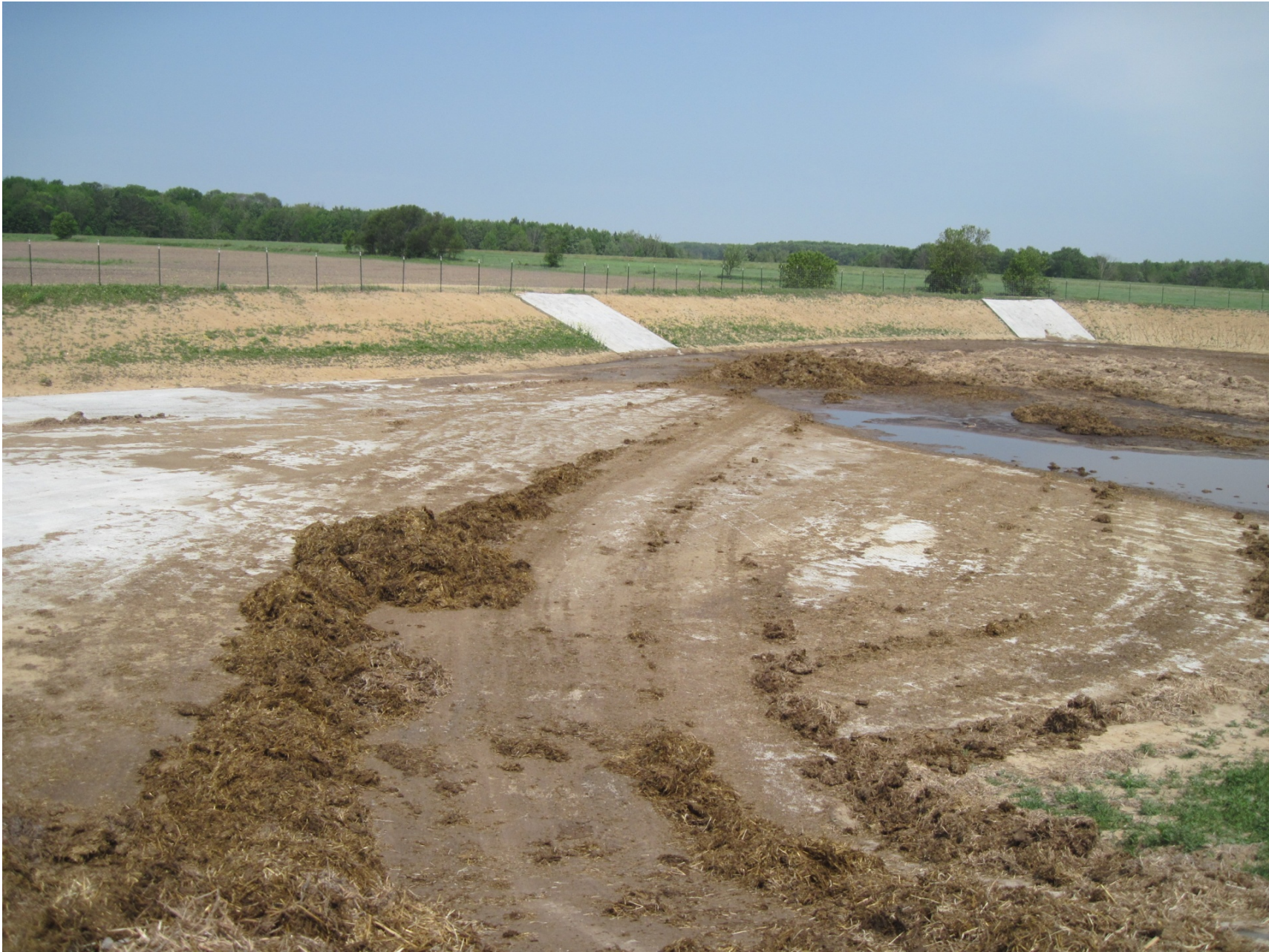
May 24, 2012 – Standing on the feedlot push-off ramp, on the southeast side of the long term manure storage facility, looking to the northwest, notice the concrete floor with earthen side slopes. The facility was emptied in spring and only had 3 months of accumulation. Fence is up and seeding on the dikes is just starting to come up.
