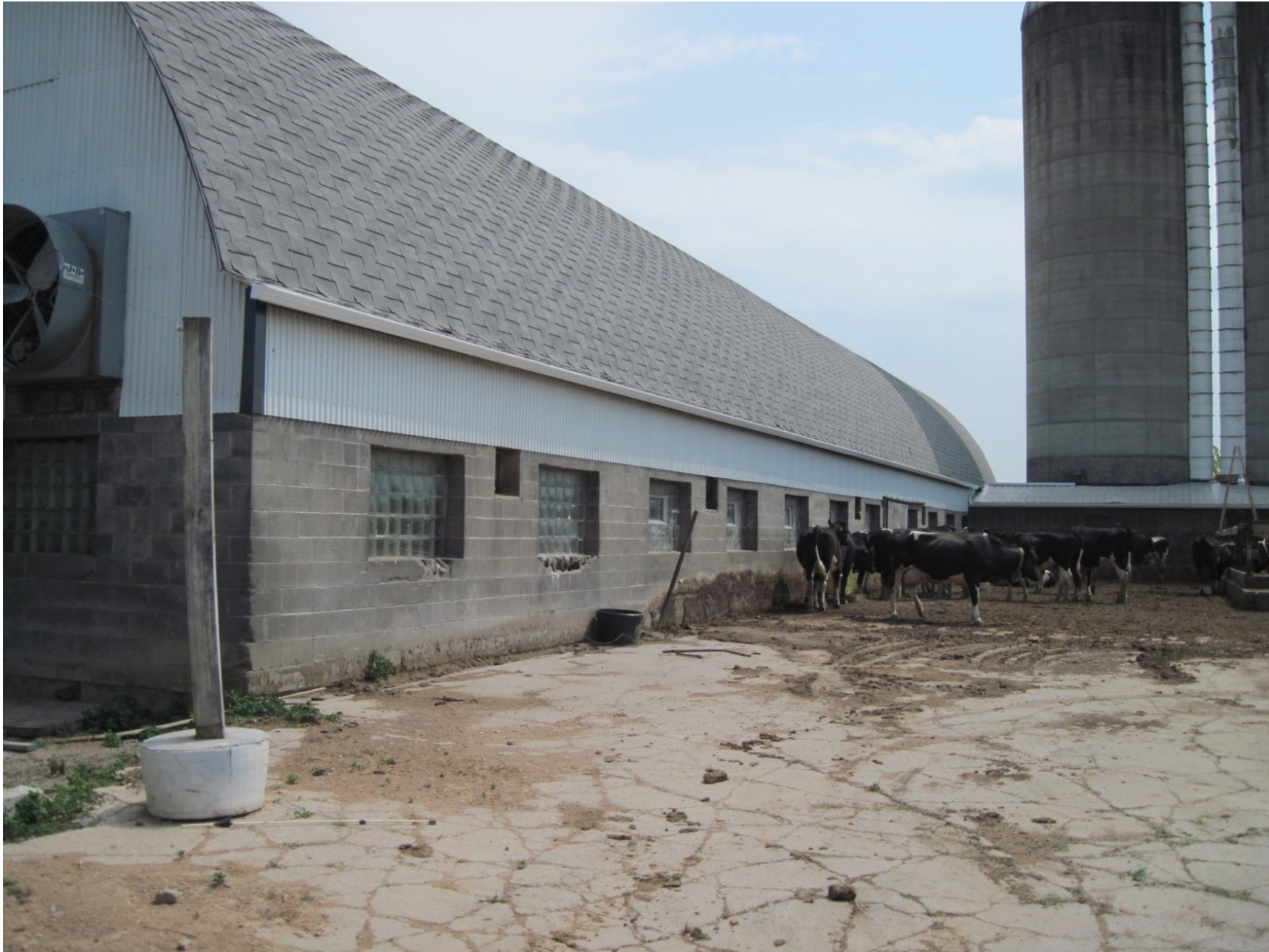
May 24, 2012 – Standing on the southwest side of the barn looking northeast over the barnyard on the south side of the barn. Since this feedlot is in a SWQMA, all clean water needs to be diverted. Roof gutters were used to catch and divert clean water.
