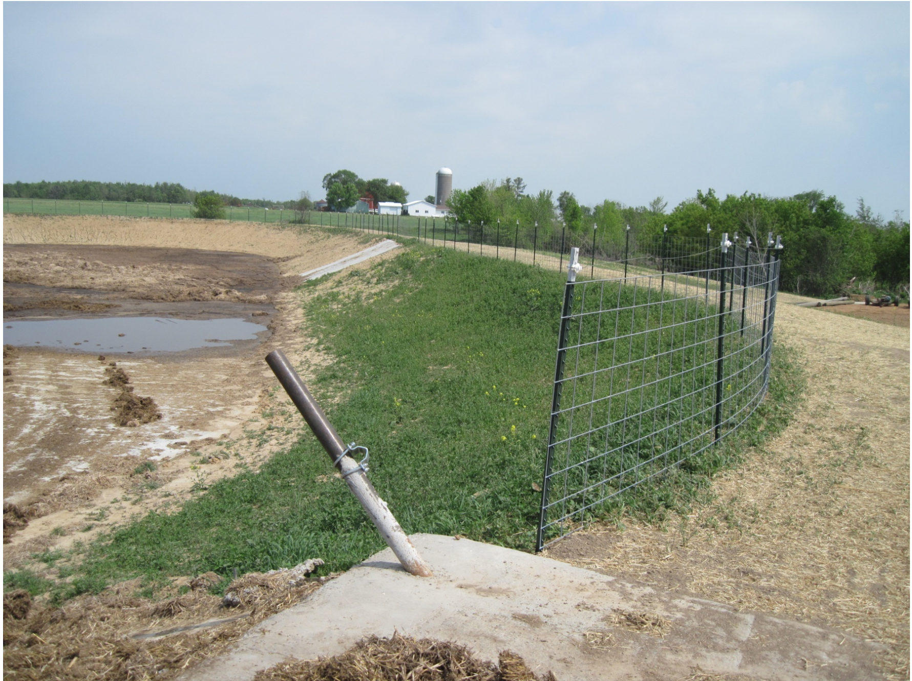
May 24, 2012 – Standing on the feedlot push-off ramp, on the southeast side of the long term manure storage facility, looking to the north along the east side of the storage. Fence is up and seeding on the dikes is just starting to come up.
