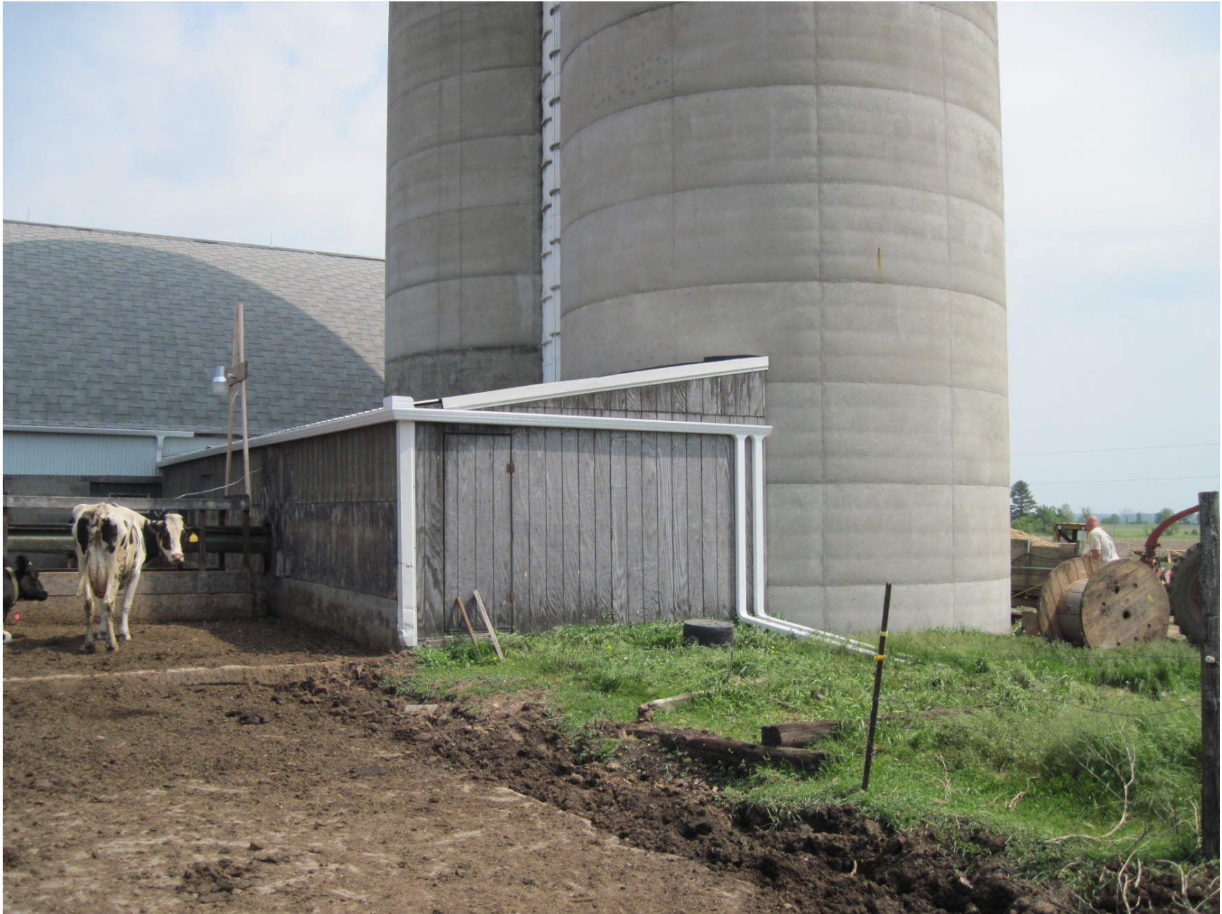
May 24, 2012 – Standing on the south side of the barn, east side of the feedlot, looking northeast, you can see that the roof gutters outlet to a stable vegetated area. Since this feedlot is in a SWQMA, all clean water needs to be diverted. Roof gutters were used to catch and divert all the roof water.
