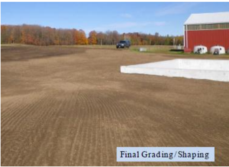
Picket Outlet for Barnyard Runoff Collection
