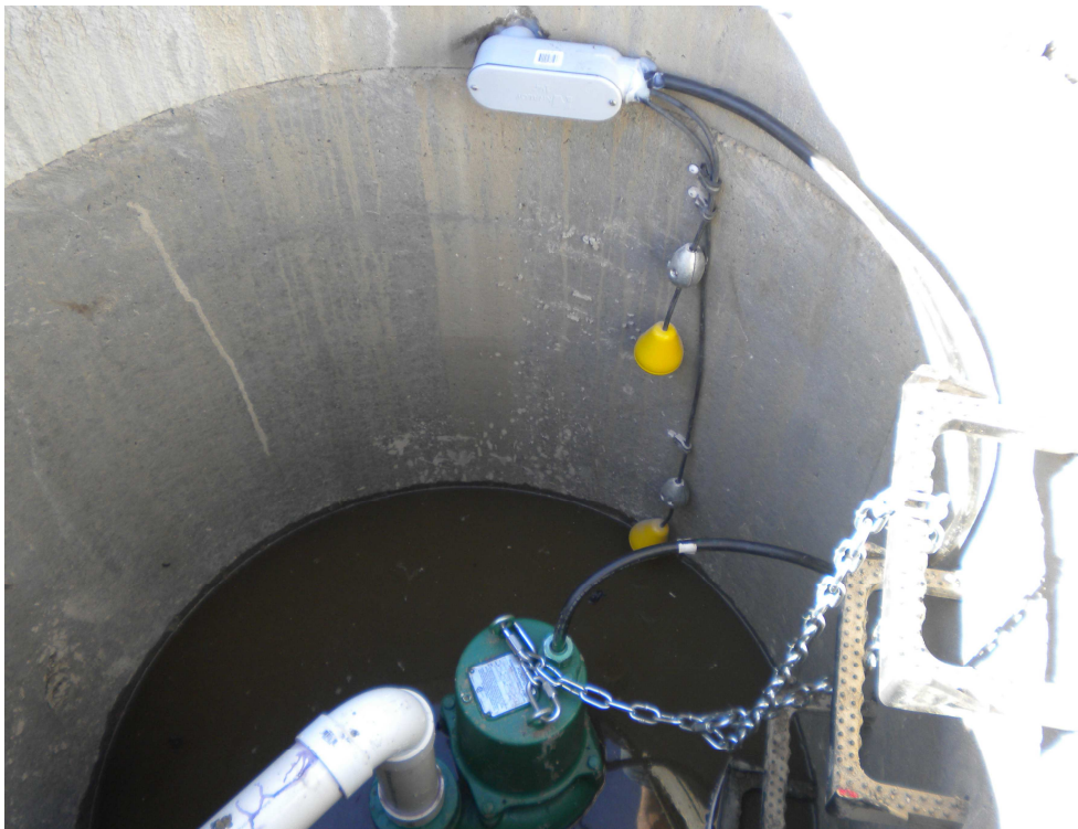
Another Picture of Barnyard Runoff Collection – Pumps to Long Term Storage Facility
