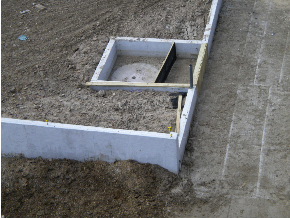
Barnyard Picket/Screens And Orifice Opening To Settle Out Manure Solids
