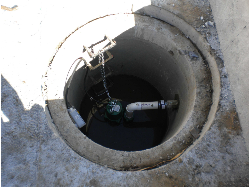
Barnyard Runoff Collection – Pumps to Long Term Storage Facility – Zero discharge
