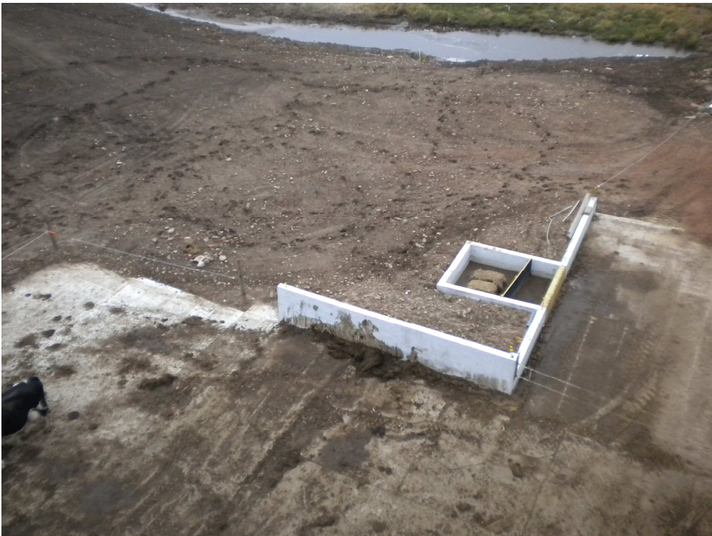
Picture of Settling Basin & Picket/Screen Assembly
