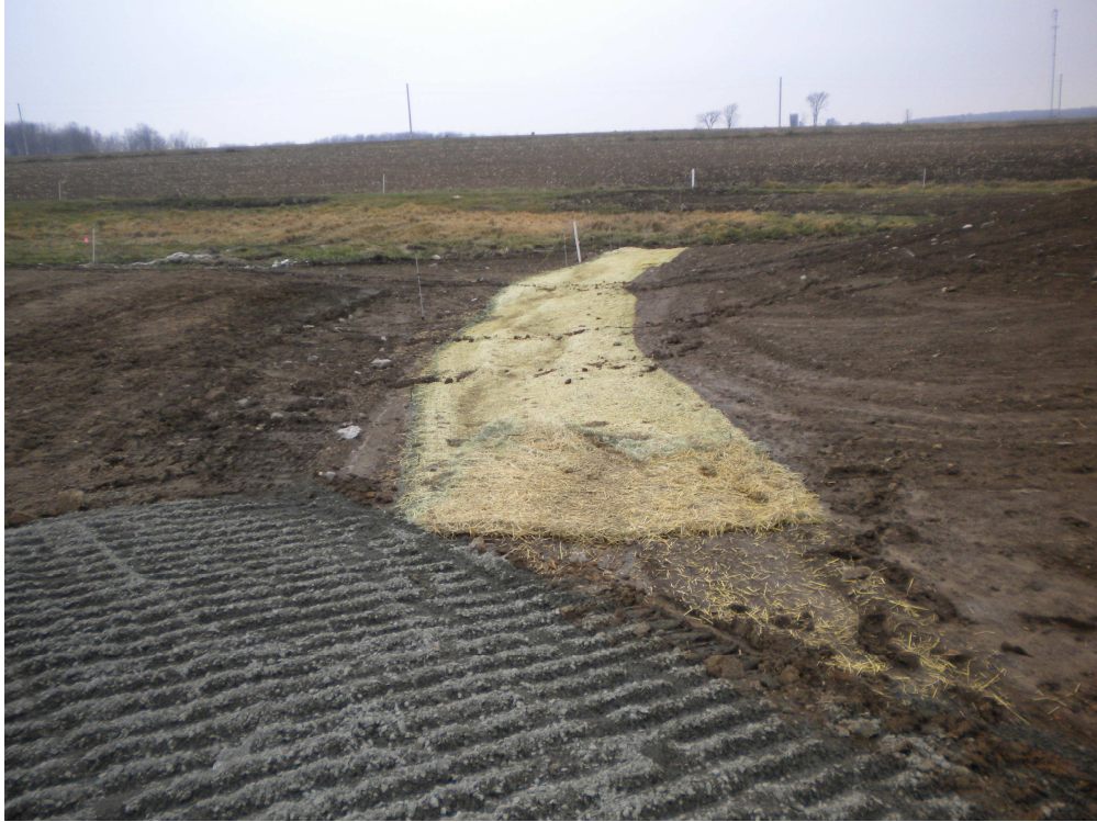
Picture of Diversion Crossing Looking Downstream Erosion Netting On Diversion Ditch
