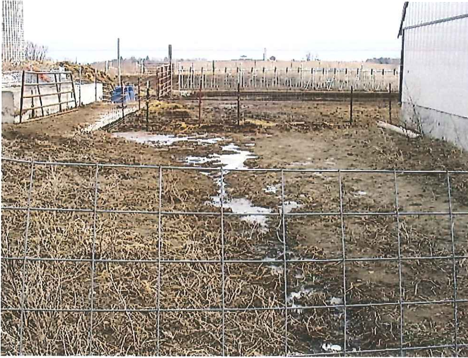
Direct discharge of concrete feedlot
