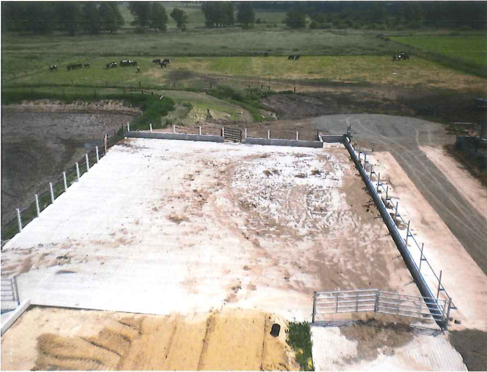
The newly constructed barnyard slopes to low corner where a sump and pump transfer waste to the waste storage facility.
