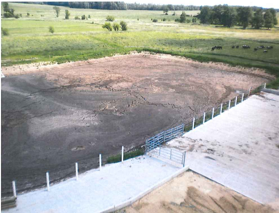
Viewing the newly constructed waste-storage facility and concrete barnyard with scrape off point from barnyard to long term storage. The pit has a clay liner.
