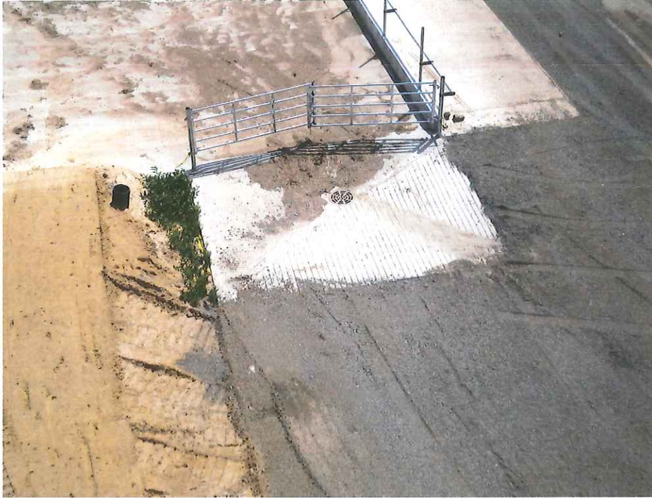
Farmstead runoff was partially redirected with a diversion ditch and the remainder of the runoff is redirected through this surface inlet and underground outlet. Clean water is transferred under the barnyard.
