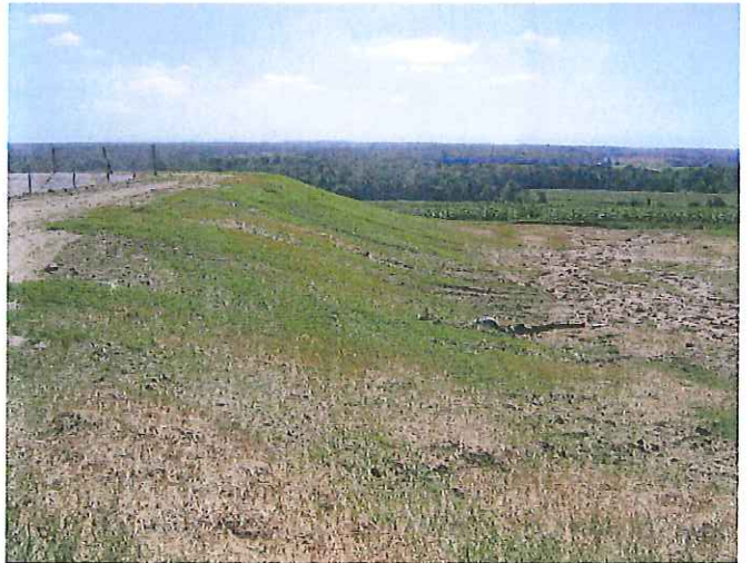
Outside berms and disturbed areas were seeded and mulch was applied to help the grow of vegetation and control erosion
