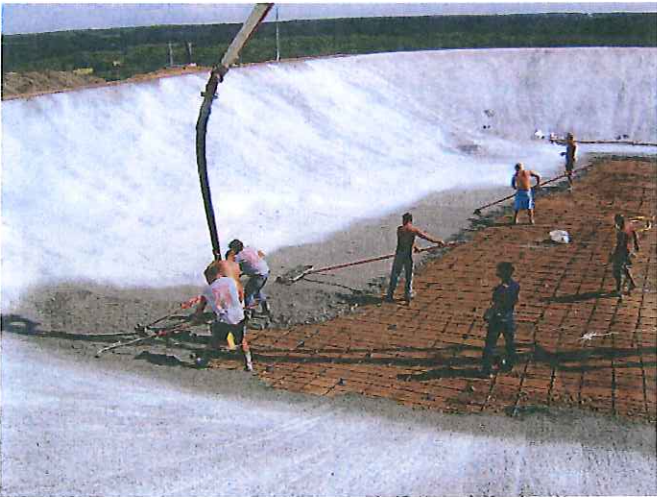
Floor concrete was installed with a pump truck, consolidated with a roller buggy and bull float. Curing compound was applied right away
