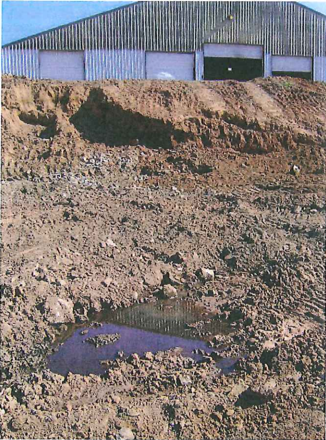
Water seepage after bedrock was hammer drilled and removed
