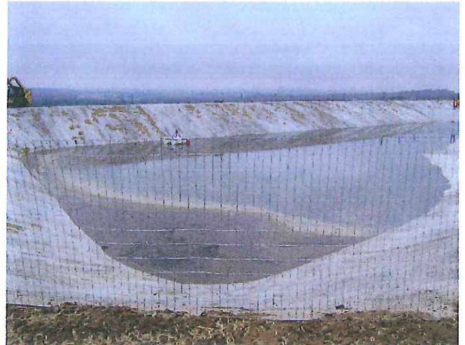
Second stage of manure storage facility with flush flume transfer collection system to transfer liquids to barn
