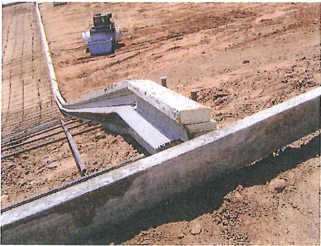
Keyway method used in forming waterstops to provide liquid joints in concrete
