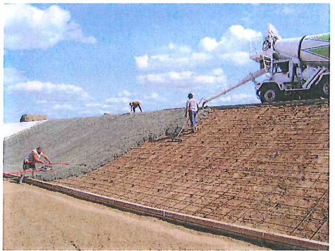
Side slopes poured with lava flow method and consolidated with roller buggy
