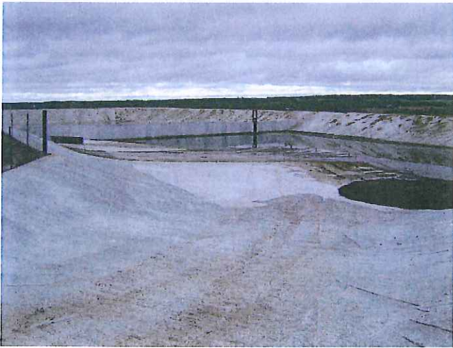
First stage of manure storage facility with flush flume transfer pipe from barn
