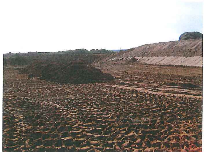
Subgrade material delivered, spread with bulldozer, and compacted with sheep's foot roller
