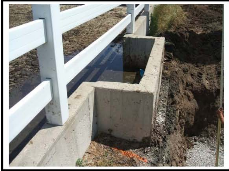
Photo #: 4 Photo Depicts: Existing barnyard runoff to filter box. Location for new tank.
