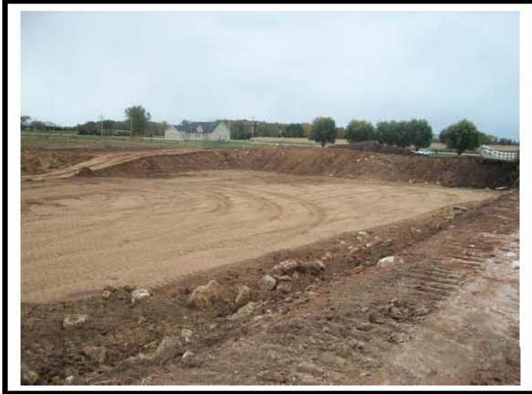
Photo #: 25 Photo Depicts: Pit construction after abandonment of existing earthen storage facility.
