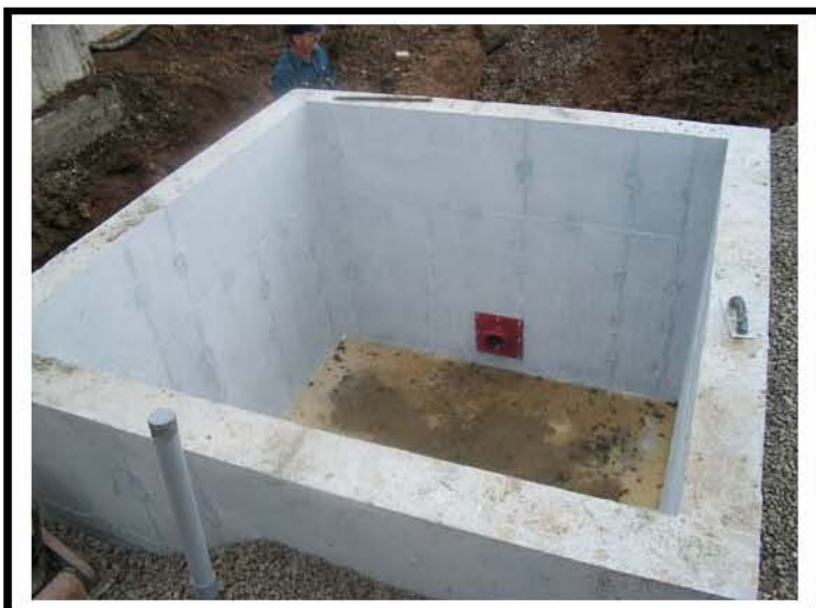
Photo #: 21 Photo Depicts: Tank construction & transfer inlet to new concrete storage facility.
