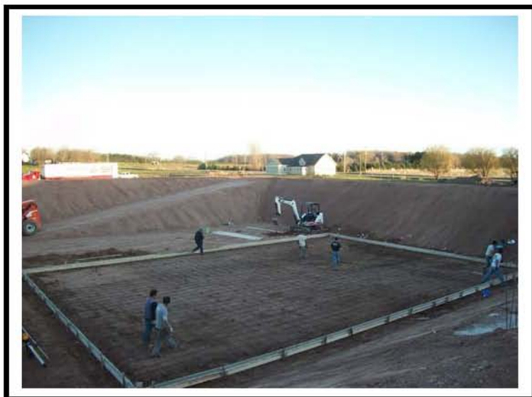
Photo #: 32 Photo Depicts: Pit construction. Forming and placing steel for first pour. Direction Pointed: Eastward
