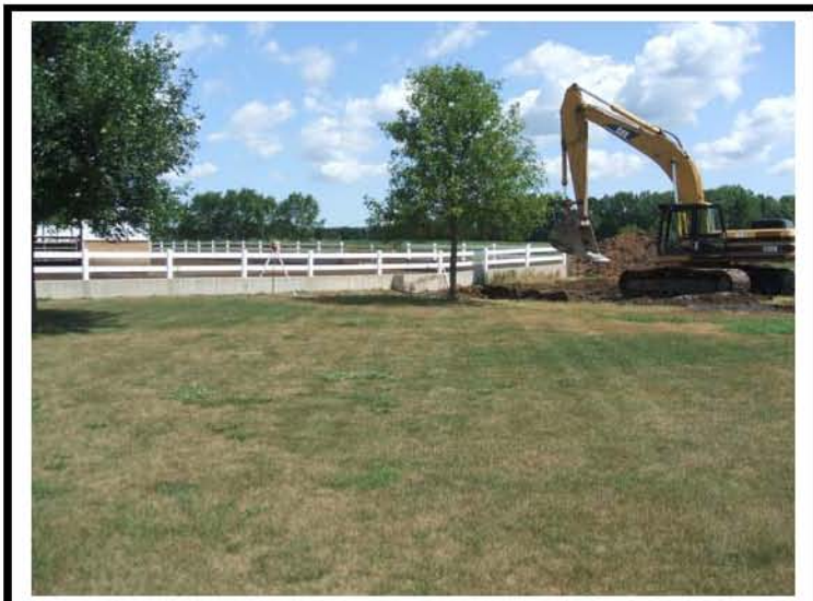
Photo #: 3 Photo Depicts: Excavation for new tank to store barnyard runoff and milkhouse waste.
