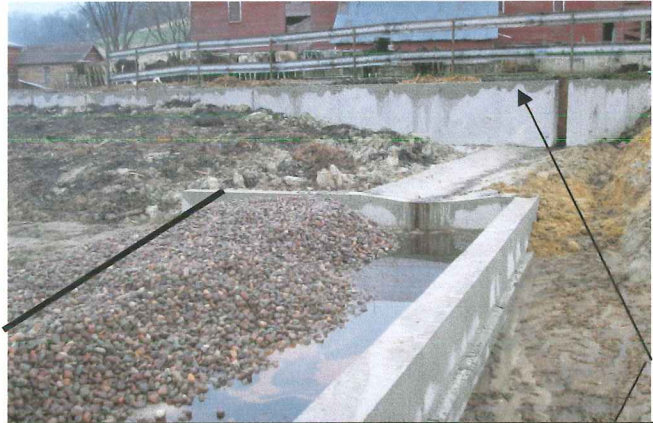
This barnyard project has an off-lot settling basin, Rock in the spreader pad will need to be pushed closer to the edge of the spreader pad, when that part of the off-lot dries out. Inside edge of the rock should be located at or close to the black line.
