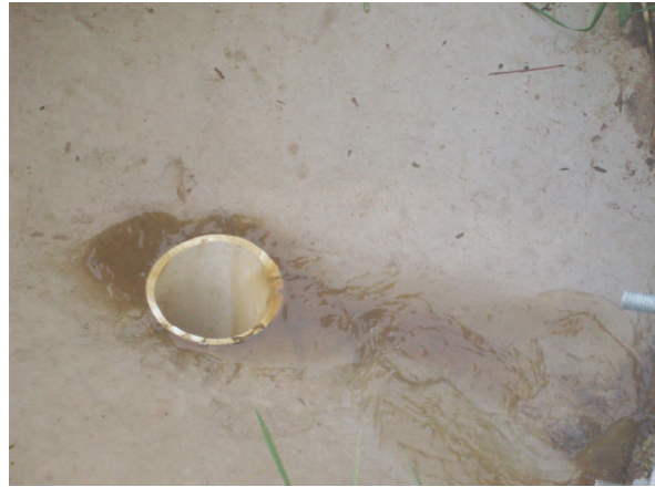
Liquids from the barnyard drop onto this concrete pad outside the barnyard walls, flow through the 4" pvc underground pipe to the filter strip (in the bottom, left photo) on the other side of the driveway.
