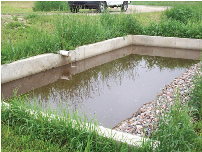
Underground pvc pipe drains to the spreader pad.
