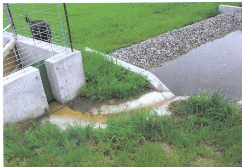
Liquids leaving the lot via weir and entering the settlement basin.
