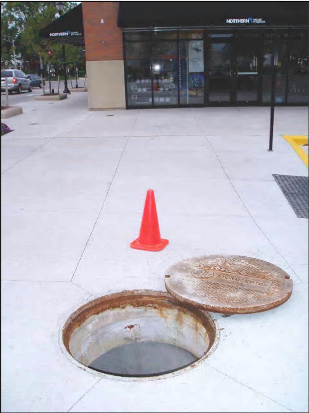
Stormceptor STC 1800 Located along Port Washington Rd on sidewalk next to Mongolian Grill
