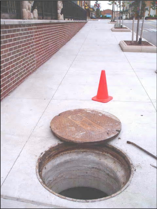
Stormceptor STC 1800 Located along Port Washington Rd on sidewalk next to Mongolian Grill
