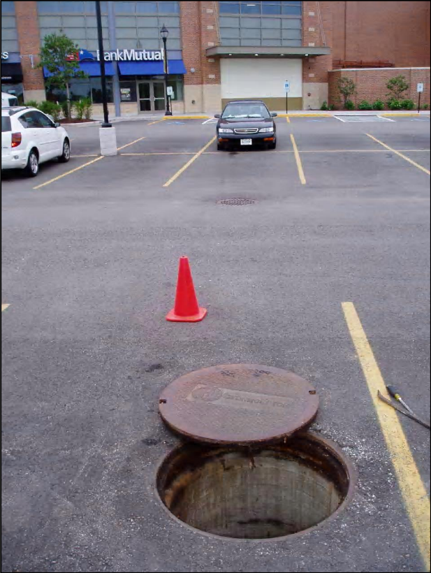
Stormceptor STC 4800 Located along Port Washington Rd in Cheesecake Factory Parking Lot
