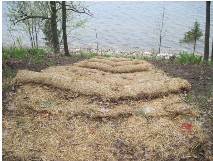
Staff from Good Oak Ecological Services perform selective tree thinning, broadcast a native woodland seed mix, and install erosion matting (Winter-Spring 2011).
