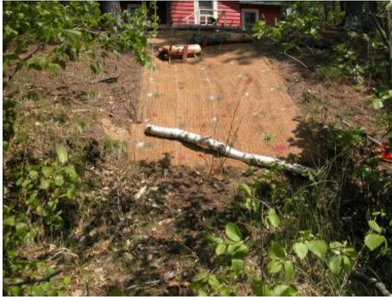
Figure 2. Coconut Erosion Control Blanket installed at Moon Beach during the summer of 2009 at moderate erosion areas (Photo by D. Haskell).
